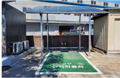
EV Charging Station using PV
