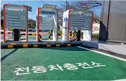
EV Charging Station
