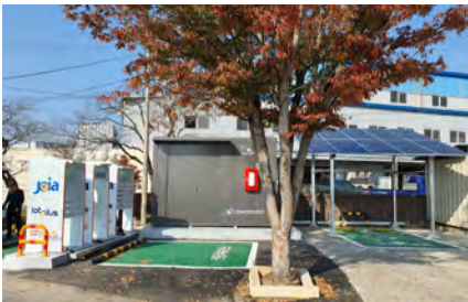
EV Charging Station & ESS
